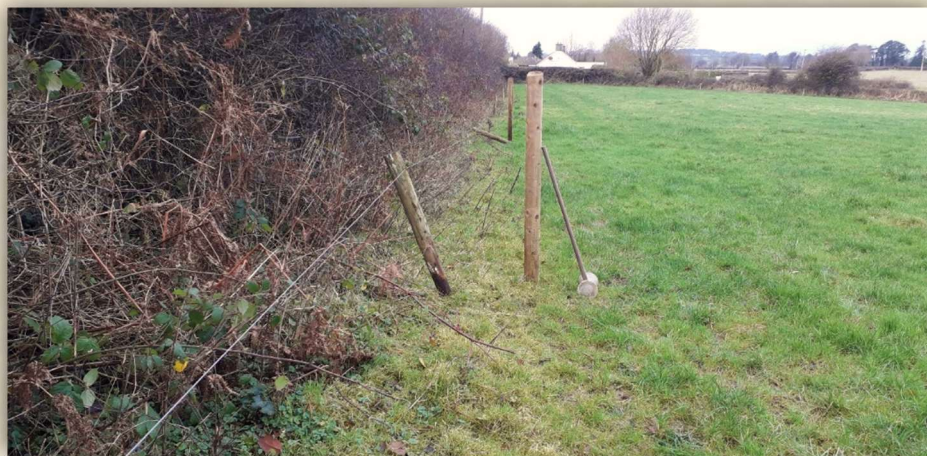
Create a field margin over time by situating new fence posts 2m from the base of the hedge
